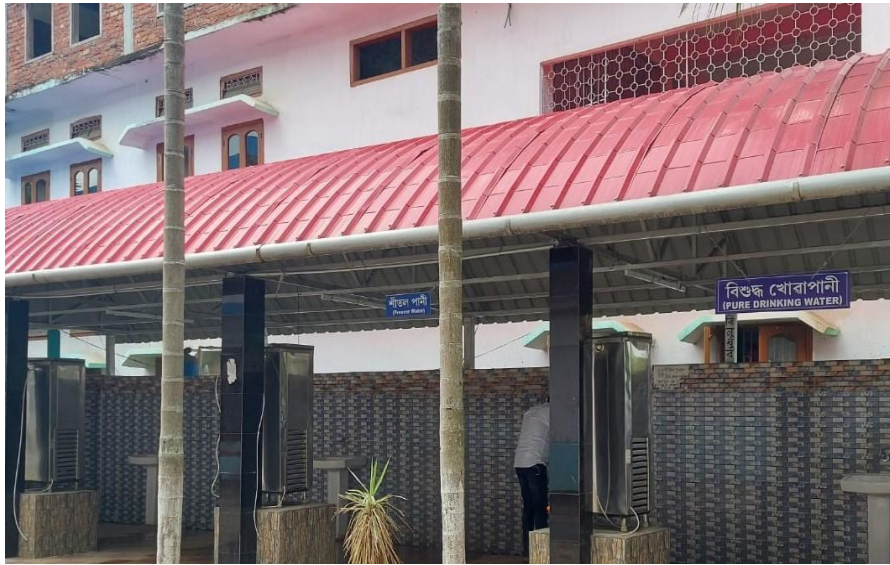
Photo 3: Water Purifiers Installed in the Campus
